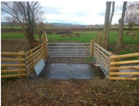
New fencing at Wernddu Farm in the Camlad catchment designed to ensure livestock doesn't enter the river that runs through the farm.
